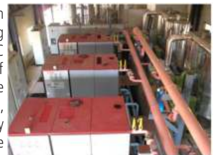
ELGI oil-free compressors at an installation
